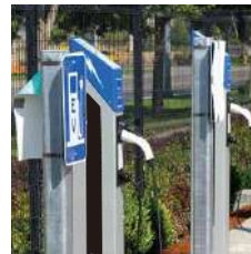
DC charging station
