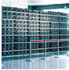
Energy storage system
